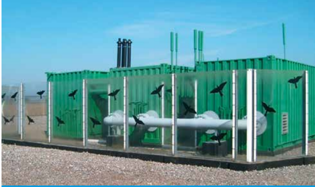
BIOGAS FEED-IN PLANT
