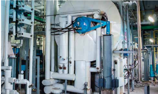
260 KT/A POLYCARBONATE POLYCONDENSATION PLANT
