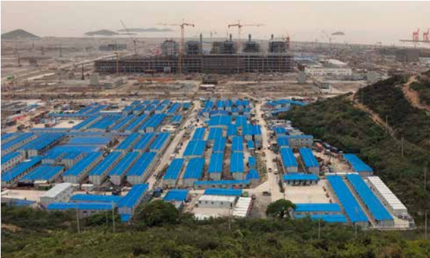
520 KT/A POLYCARBONATE POLYCONDENSATION PLANT
