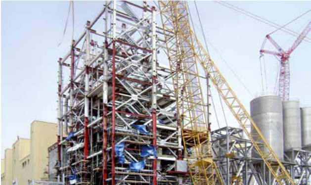
REVAMPING OF 4 EXISTING POLYCONDENSATION PLANTS
